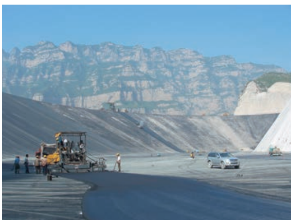
Xilongchi Pumped-storage Power Station in China
